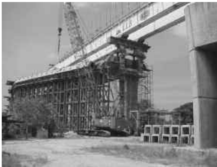
Figure 9: Construction of bifurcation using combination of launching gantry and heavy duty falsework
